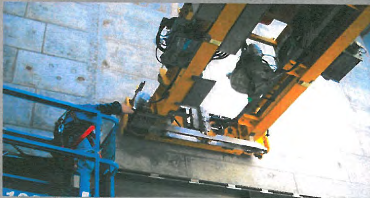
High-Level Waste Facility bridge crane
