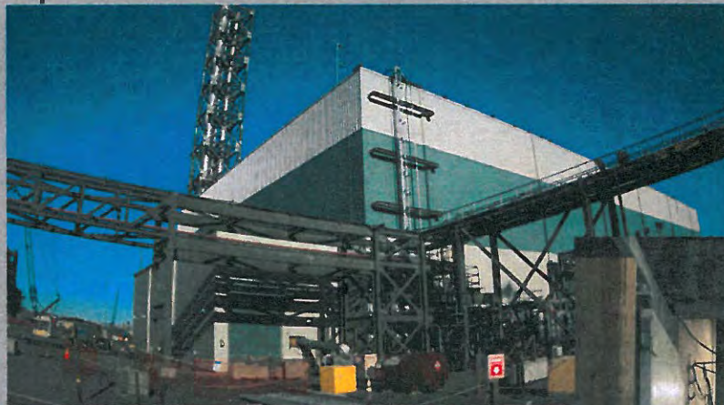
Overhead pipe racks for steam and glass-formers
