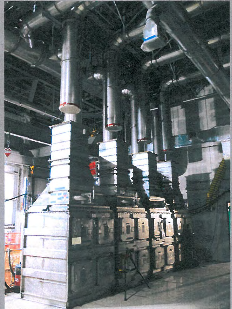
Analytical Laboratory air-handling systems
