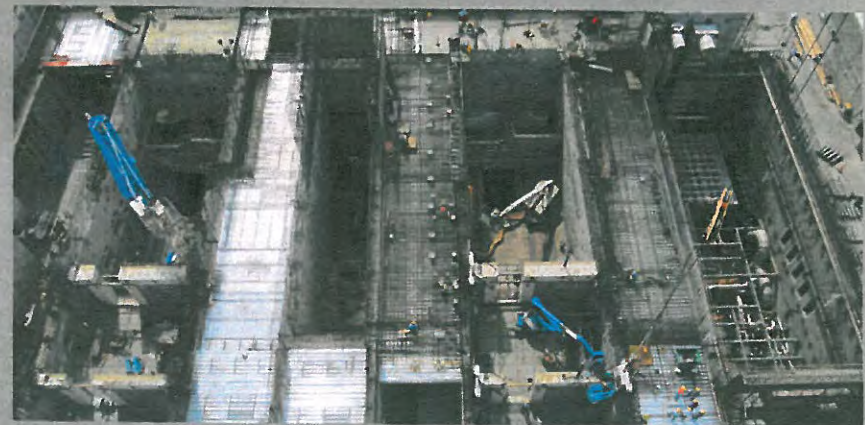
High-Level Waste Facility melter bay
