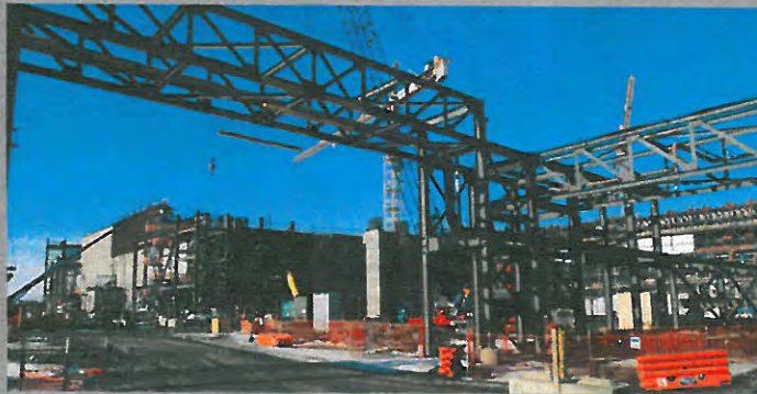
Overhead pipe racks for steam and glass-forming materials
