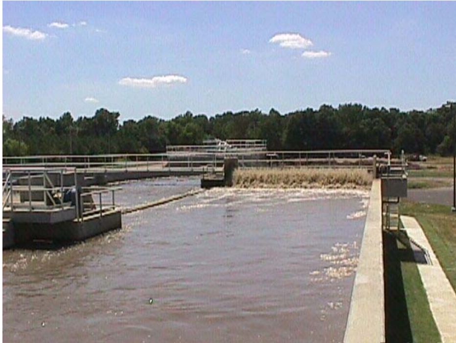
Figure 2: Oxidation Ditch/Aeration Rotor at the City of Bartlett WWTP #1 (Photo provided courtesy of the City of Bartlett Wastewater Division)
