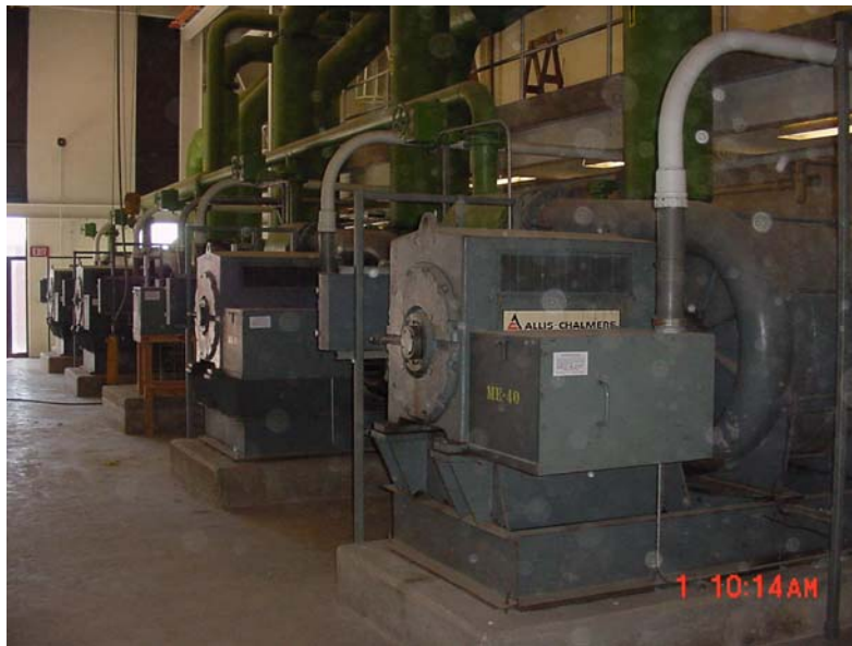
Figure 3: Multi-stage Centrifugal Blowers - GBMSD - De Pere Wastewater Treatment Facility (Photo provided courtesy of the Green Bay Metropolitan Sewerage District)
