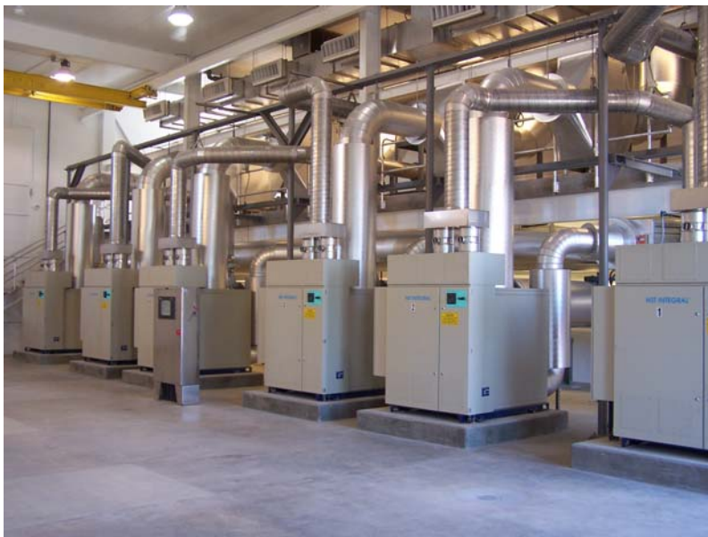
Figure 4: Magnetic Bearing Turbo Blowers - GBMSD - De Pere Wastewater Treatment Facility (Photo provided courtesy of the Green Bay Metropolitan Sewerage District)
