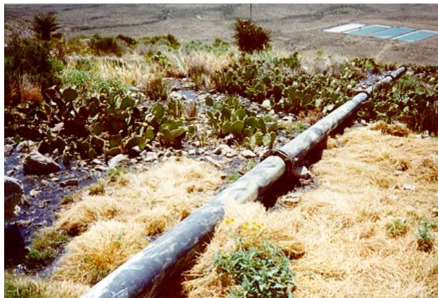
Main sewer line leak discovered in early June, 1998. Sewage is flowing from left of photo. Note sewage lagoons in the background. (NPS Photo by Dale Pate)
