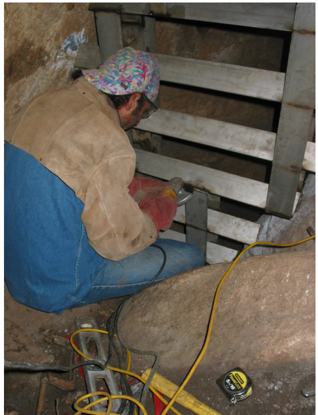
Charlie Savas of Zara Environmental welds a new gate in place on the main entrance to Soldiers Cave. Park staff hopes this gate is more bat and wildlife friendly, and more secure to help protect this delicate cave.
