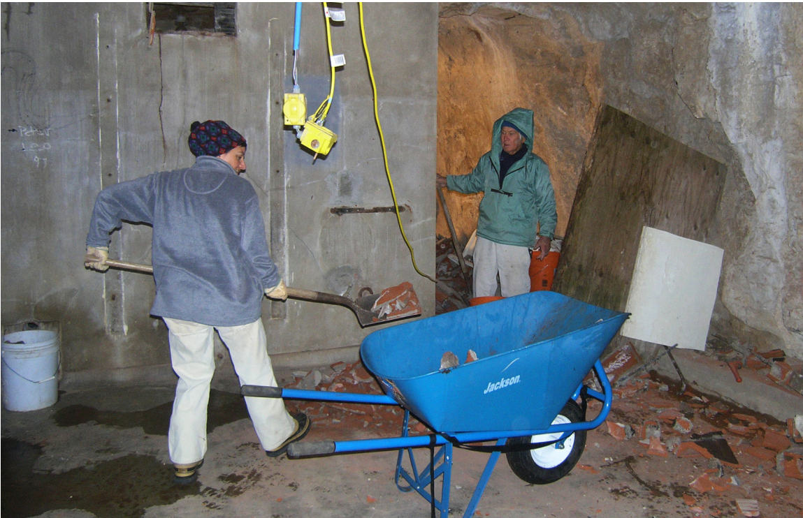
Barbara Ruble and Vance Nelson, volunteers from the Western Region of the NSS, work to remove rubble from the demolished and abandoned Crystal Cave restrooms inside Crystal Cave in Sequoia National Park. This work was part of this year's annual Crystal Cave Restoration held October 23 through 31. More than 300 wheel barrow loads of this debris were moved 1/2 mile to the Crystal Cave parking lot during the restoration.
