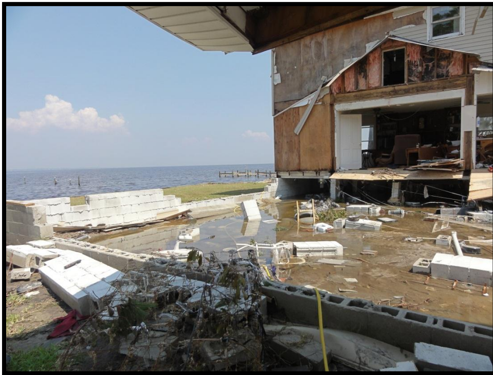
Figure. Home destroyed near Jarvis Landing
