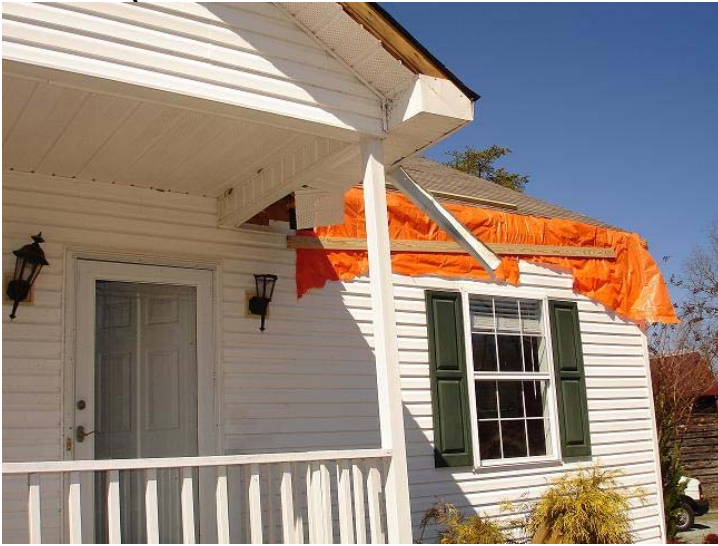
Photo 1 (House on Willie Pace Road – Porch and eave damage)
