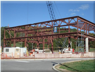
MAXLAB construction site in late October as seen from Bethel Valley Road.
