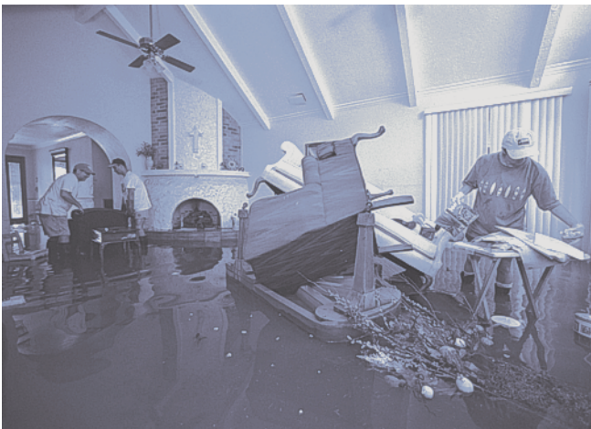
Tropical Storm Allison Damage Photo: © Houston Chronicle
