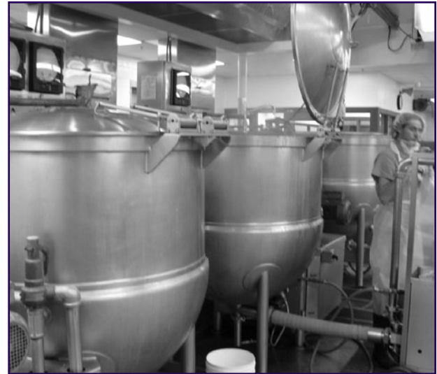
Cook-chill cooking and bagging system.
