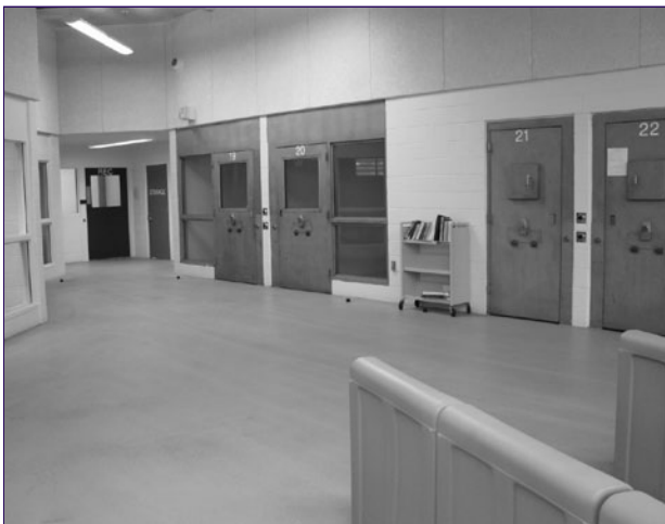
An acute medical unit with mental health cells. Note the security doors and large windows into the individual cells. (Photograph courtesy of Voorhis Robertson Justice Services.)
