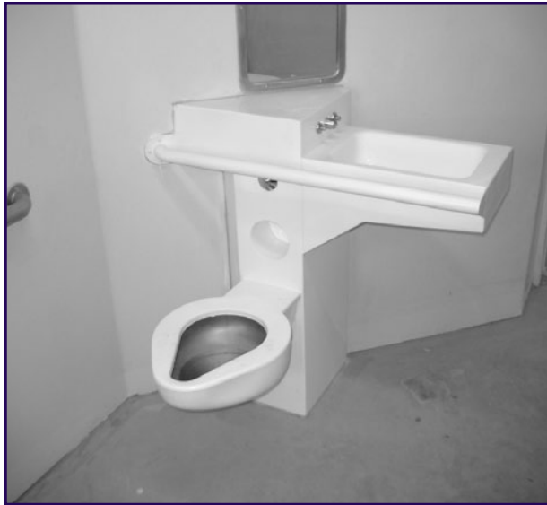
Specially designed toilet and sink combination unit with grab bars for use by inmates with disabilities. (Photograph courtesy of Liebert & Associates.)
