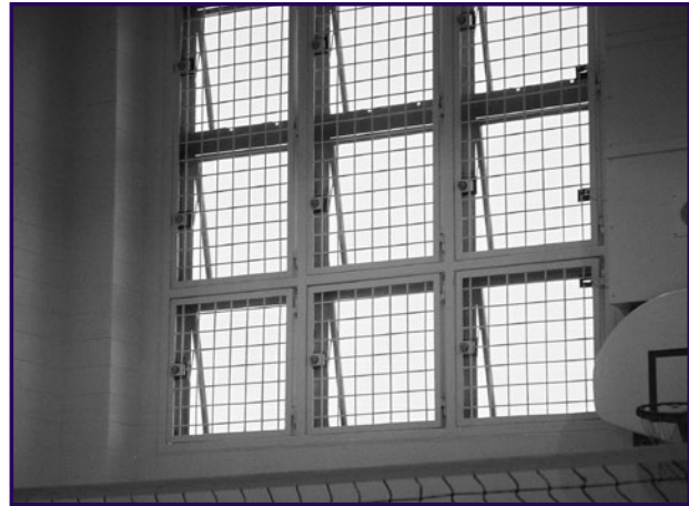
Secured windows in an indoor recreation yard. Note that these windows open for air circulation but have security mesh to prevent penetration. (Photograph courtesy of Voorhis Robertson Justice Services.)
