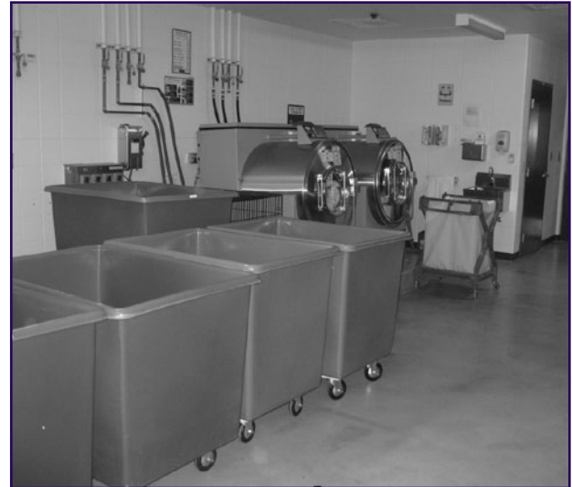
Washers in a new laundry area with enough room to store laundry collection bins.
