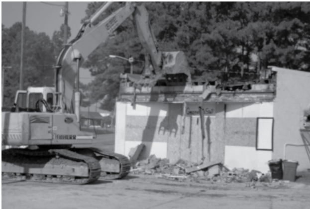
(1) Store in Greenville, NC being demolished to prevent the possibility of illegal activities resuming at the site. Greenville, NC Police Department Photo.
