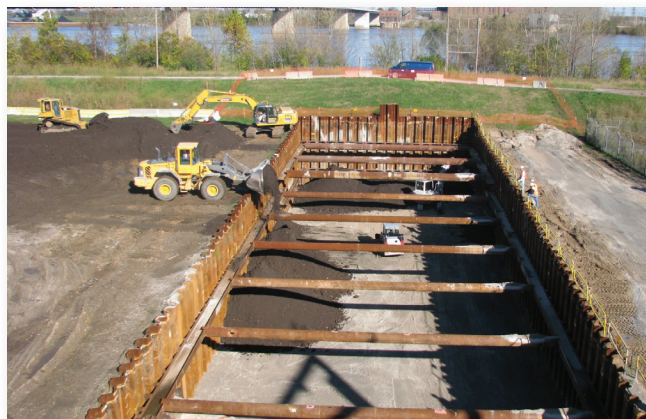
In FY09, the USACE initiated excavation west of the flood protection levee at City Property (DT-2).
