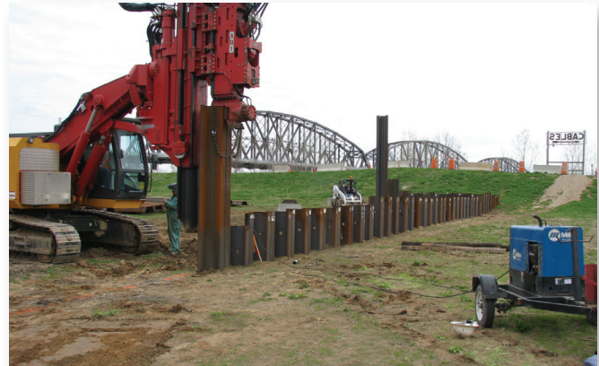
Heavy pile-driving equipment is used to initiate the sheet pile protection for the City Property Vicinity Property at SLDS.
