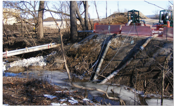
Two large pumps divert Coldwater Creek flow around an excavation at the Norfolk Southern Vicinity Property in North County.
