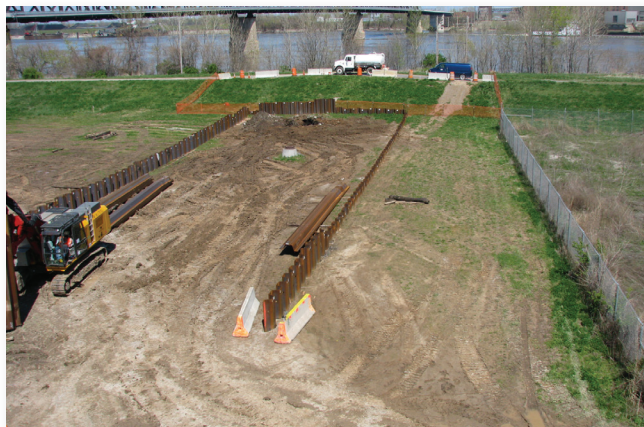
Sheet pile protection system for the City Property excavation is shown nearing completion.
