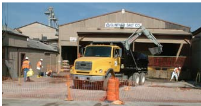
Excavation activities at Gunther Salt North and South resulted in the removal of 2,826 cy of contaminated material to an out-of-state licensed/permitted disposal facility.
