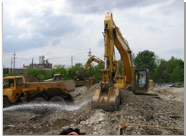
Excavation activities have begun in Phase 4 and 5 on the western border of SLAPS.
