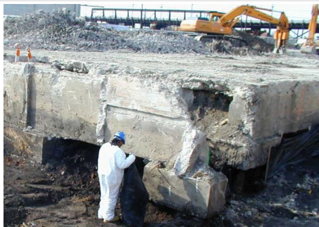
Nearly 23,000 cubic yards of contaminated soil and debris have been removed from the 4.5-acre Plant 6 East Half since December 2000.
