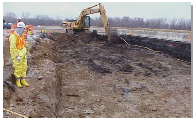
Workers finished the McDonnell Boulevard drainage ditch before spring rains impacted work.
