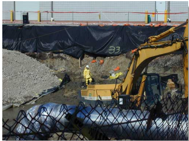
Excavation of Plant 2 concluded in April with the removal of approximately 10,200 cubic yards of material.
