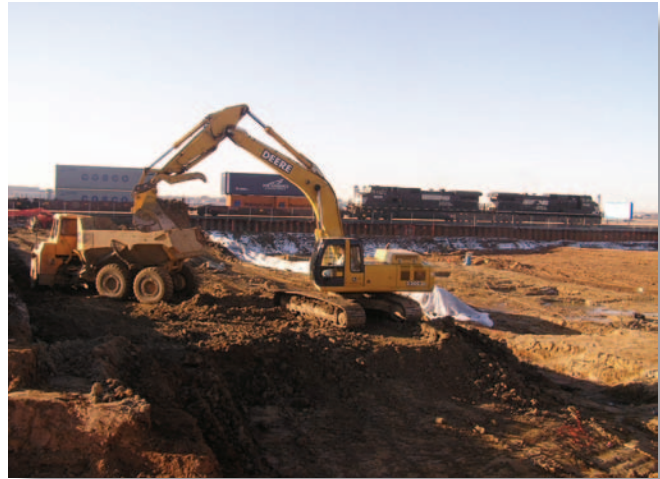
To position the site for completion in 2007, SLAPS contaminated soils will be stockpiled onsite beside the railcar loading area.
