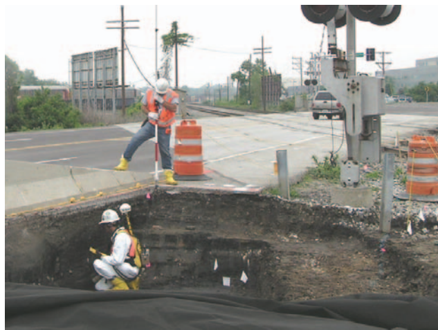
USACE closely coordinated its field activities with local agencies and utilities to support Norfolk Southern Rail Line's crossing signal replacement project.
