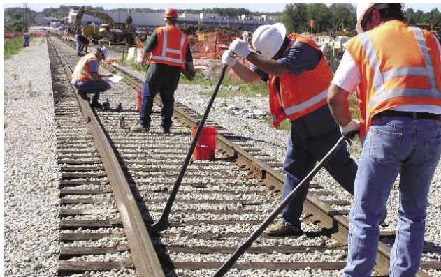
Crews relocated the SLAPS rail load out facility to facilitate completion of the final phase of cleanup at the site.
