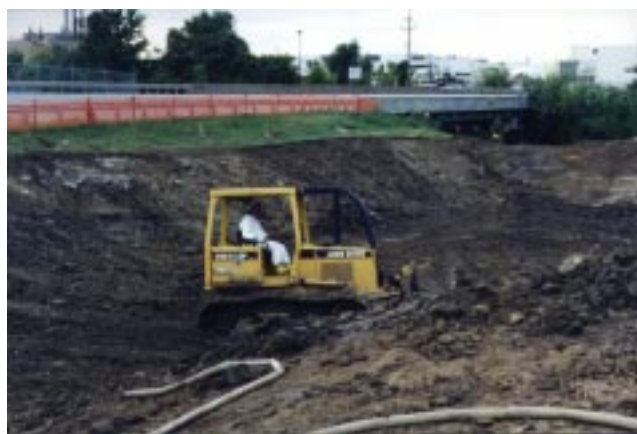
The USACE constructed a sedimentation trap to manage runoff north of McDonnell Boulevard.
