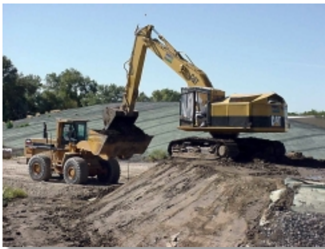
The excavator (shown above) is moving material from the HISS Supplemental Pile into a front end loader, which takes the material directly to the railcars.
