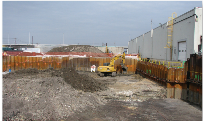
The final phase of cleanup on Mallinckrodt's Plant 6 West Half is well underway. Sheet piling forms walls around the excavation.
