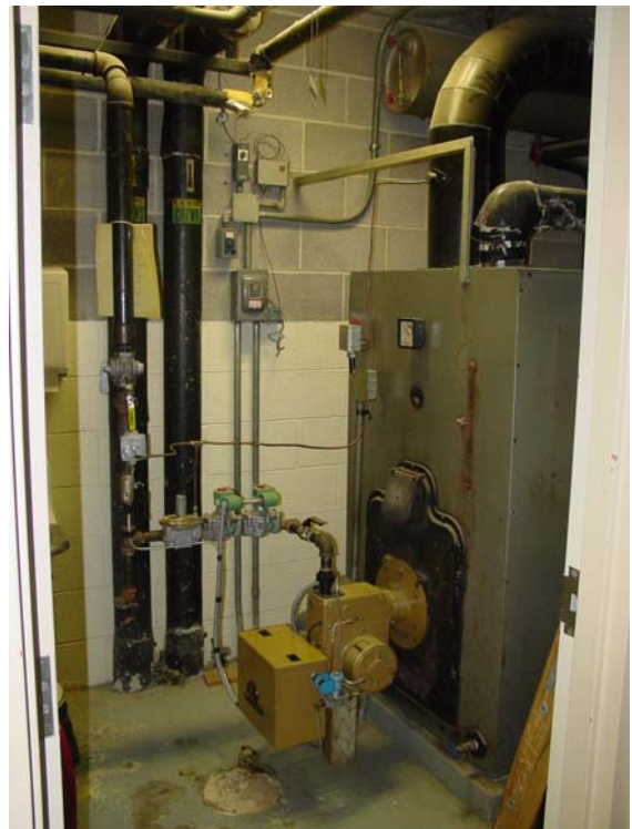
Heating and Cooling Boiler System is not energy efficient
