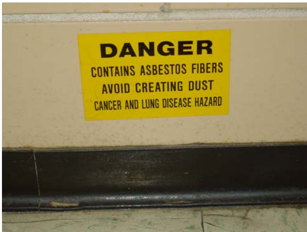
Asbestos is present
