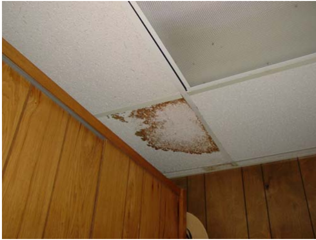
Evidence of leaking roof is present throughout the Administration Building
