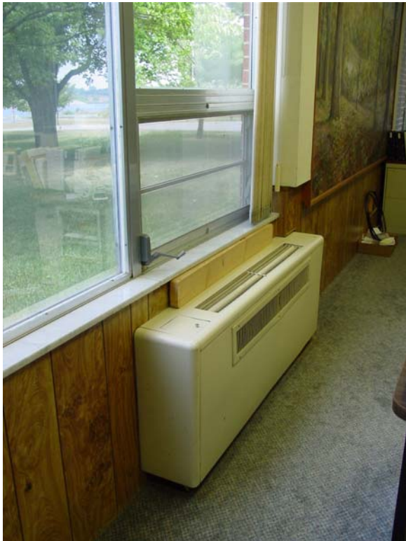
Heating and Cooling Unit
