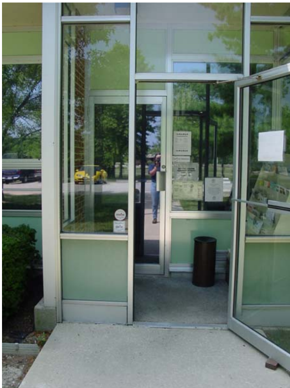
Front Entrance Doors Do Not Meet Uniform Federal Accessibility Standards (UFAS)
