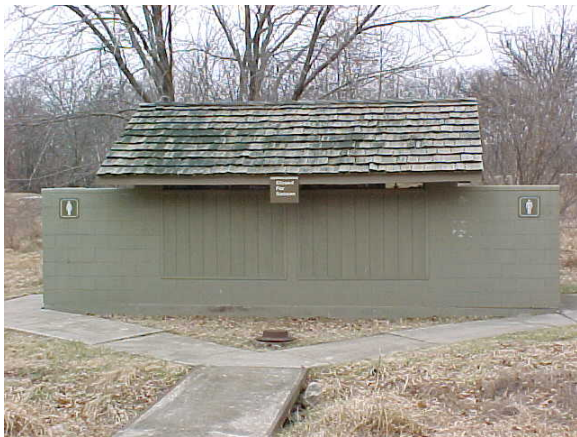
Comfort Station #3 has been removed and will be replaced with mini-shower building within Walleye Group Camp
