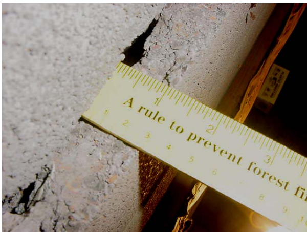
Wall Crack Movement Measurement
