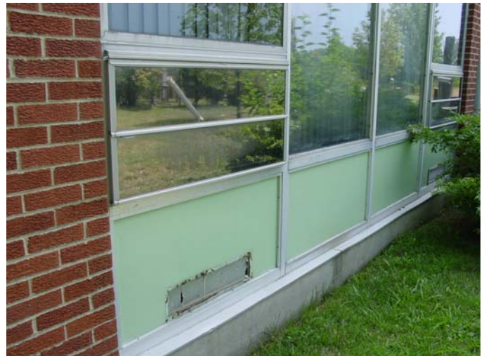
Windows are inefficient
