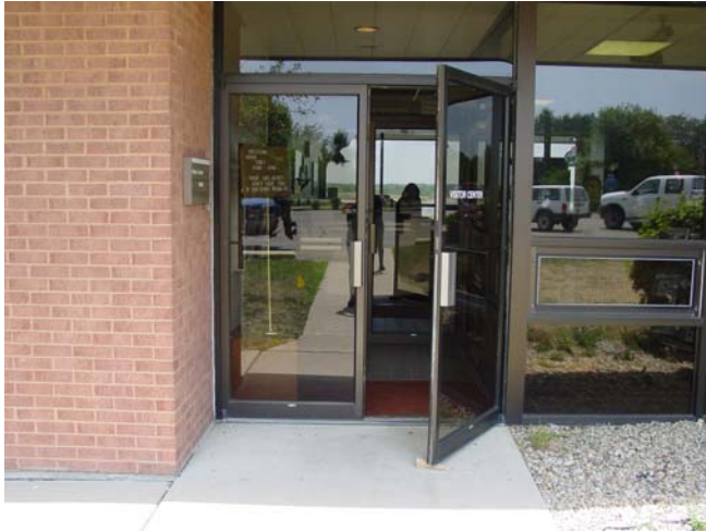
Front entrance doors do not meet Uniform Federal Accessibility Standards
