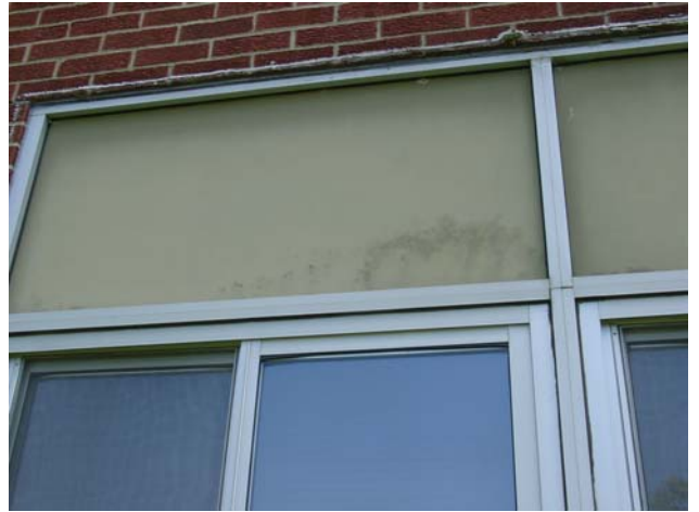
Moisture is Infiltrating in and around the Window Frames
