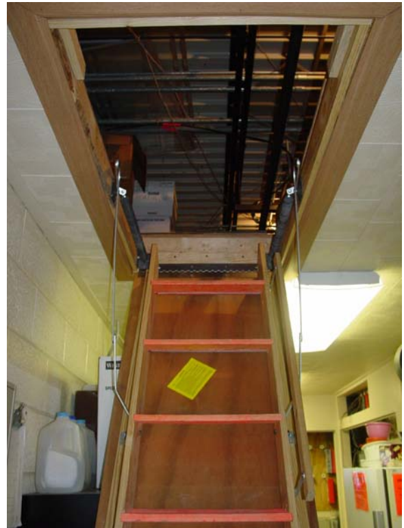
Attic used as storage area – Pull down Ladder is used to access the attic
