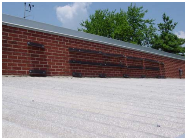
Temporary Fix for Cracked Wall
