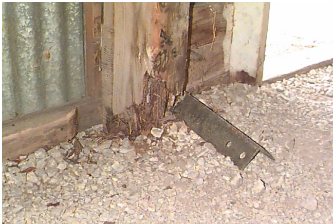
One of the main support beams in the Groves Building that is deteriorated at base
