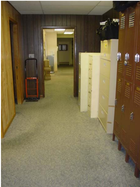
Main Hallway used as Storage Area
