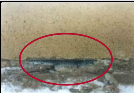
Fold lath metal and place in holes in the foundation of houses
