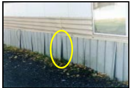
Fix gaps in trailer skirtings
