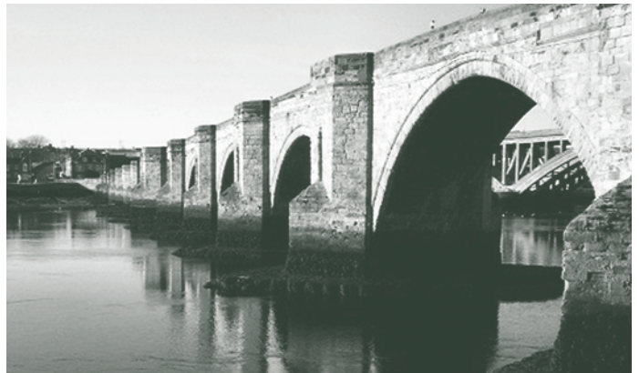
Figure 4. Similar to other countries, England has significant challenges maintaining the condition of historic bridges.
