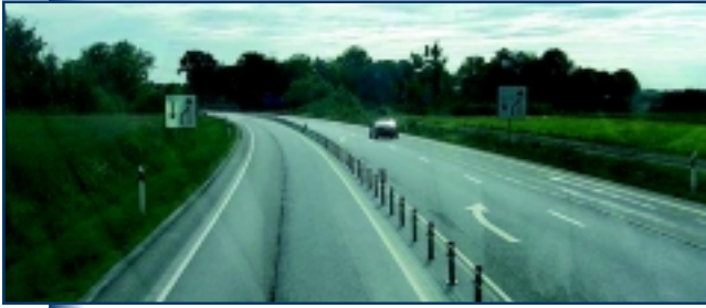
Figure 10. Use of cable barrier in 2+1 road, Sweden.
