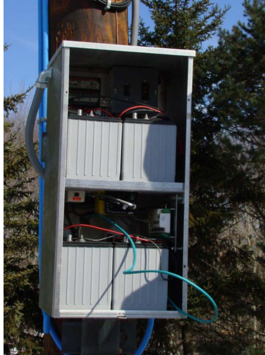
Figure 9. Batteries Used to Store Power from Solar Panels
