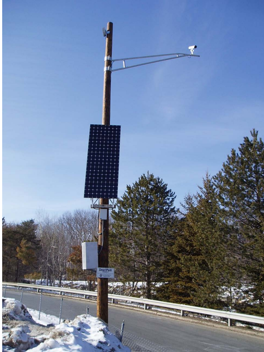
Figure 8. Inbound Pole Showing (from bottom) Ethernet Radio, Solar Battery Power Unit (SBPU), and Video Camera
