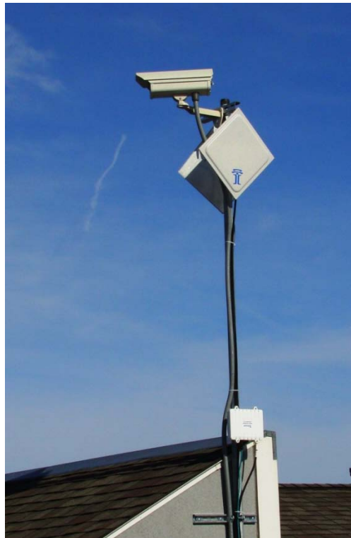
Figure 12. Single Roof-Mounted Ethernet Camera, Radio, and Directional Antennas
