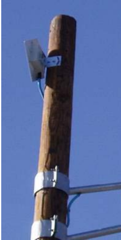
Figure 11. Pole-Mounted Ethernet Radio with Directional Antenna
