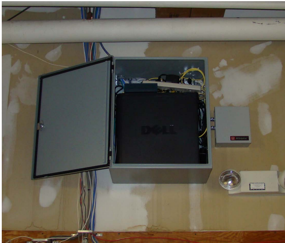
Figure 13. The Onsite Computer Mounted in the Electrical Room
