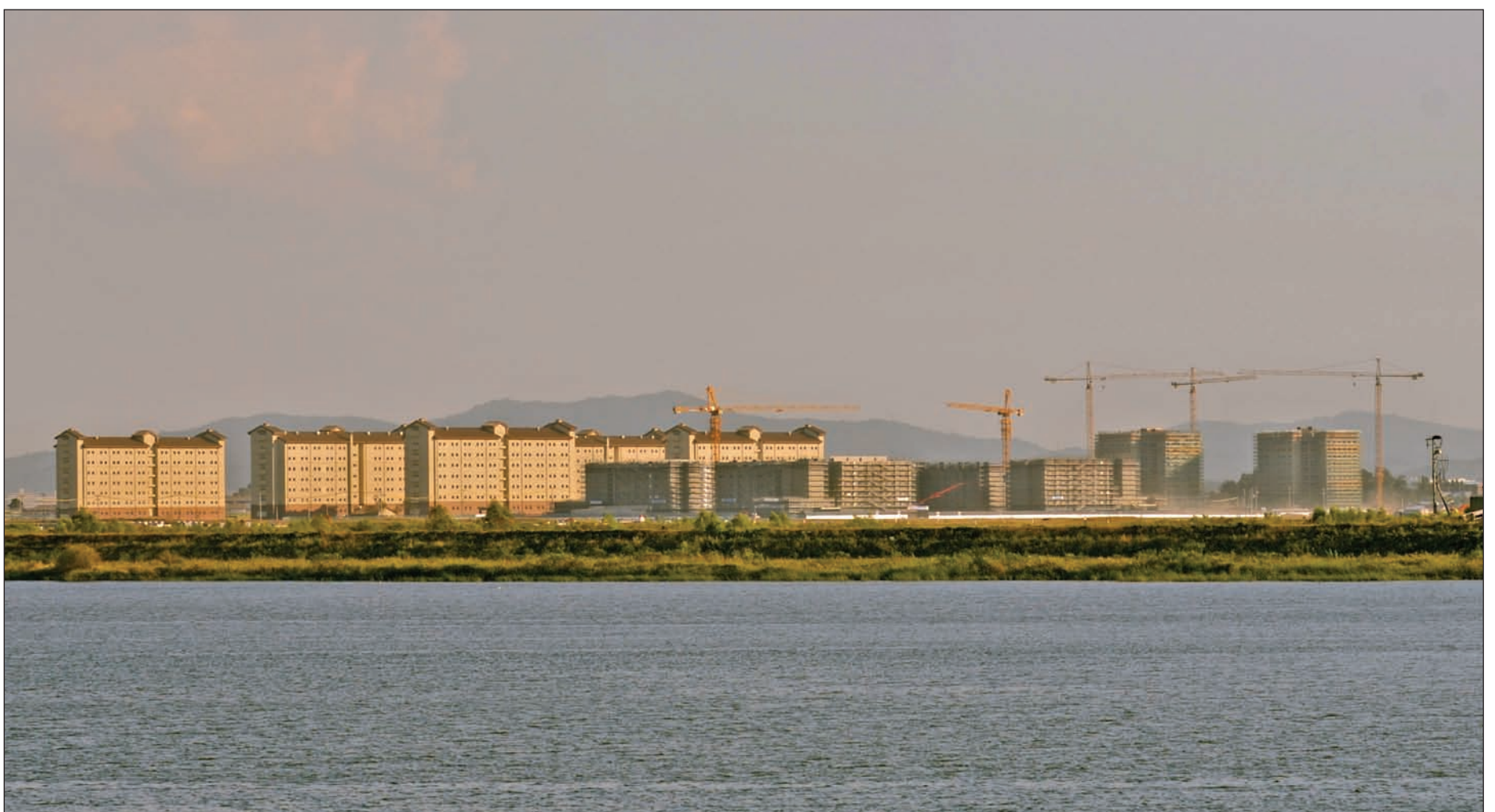
The largest construction project in the history of the Department of Defense is underway on Camp Humphreys. Building new living quarters for families and single Soldiers is a command priority as U.S. Forces Korea prepares to move from Seoul, and areas north of the city, to Camp Humphreys. Housing units like those pictured here, under construction on Camp Humphreys, are designed to give Soldiers and families a sense of normalcy and community with every modern amenity one would expect to find in the States while living overseas. — U.S. Army photo by Edward N. Johnson
