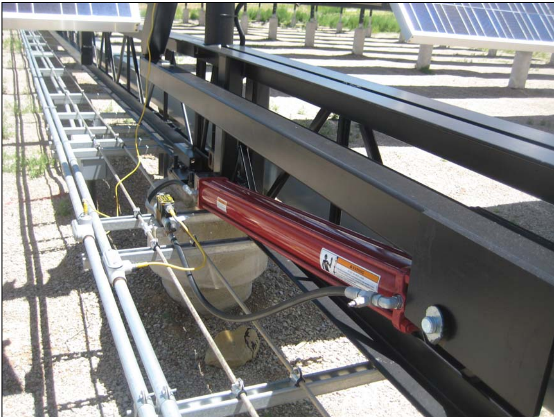
Figure 8: Example of a Tracking Solar PV Installation
