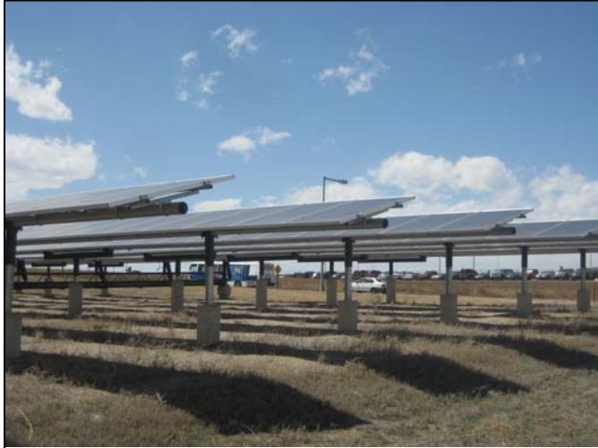
Tracking system at the Pena Boulevard Solar Farm
