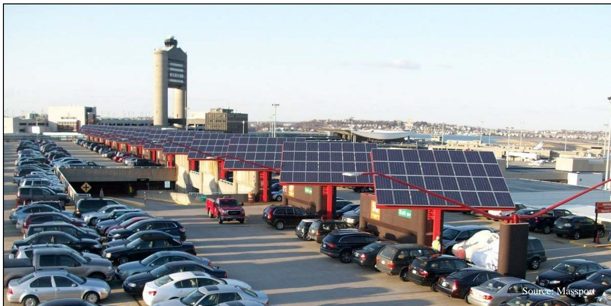
Figure 21: Solar Trees on Parking Garage at Boston's Logan Airport
