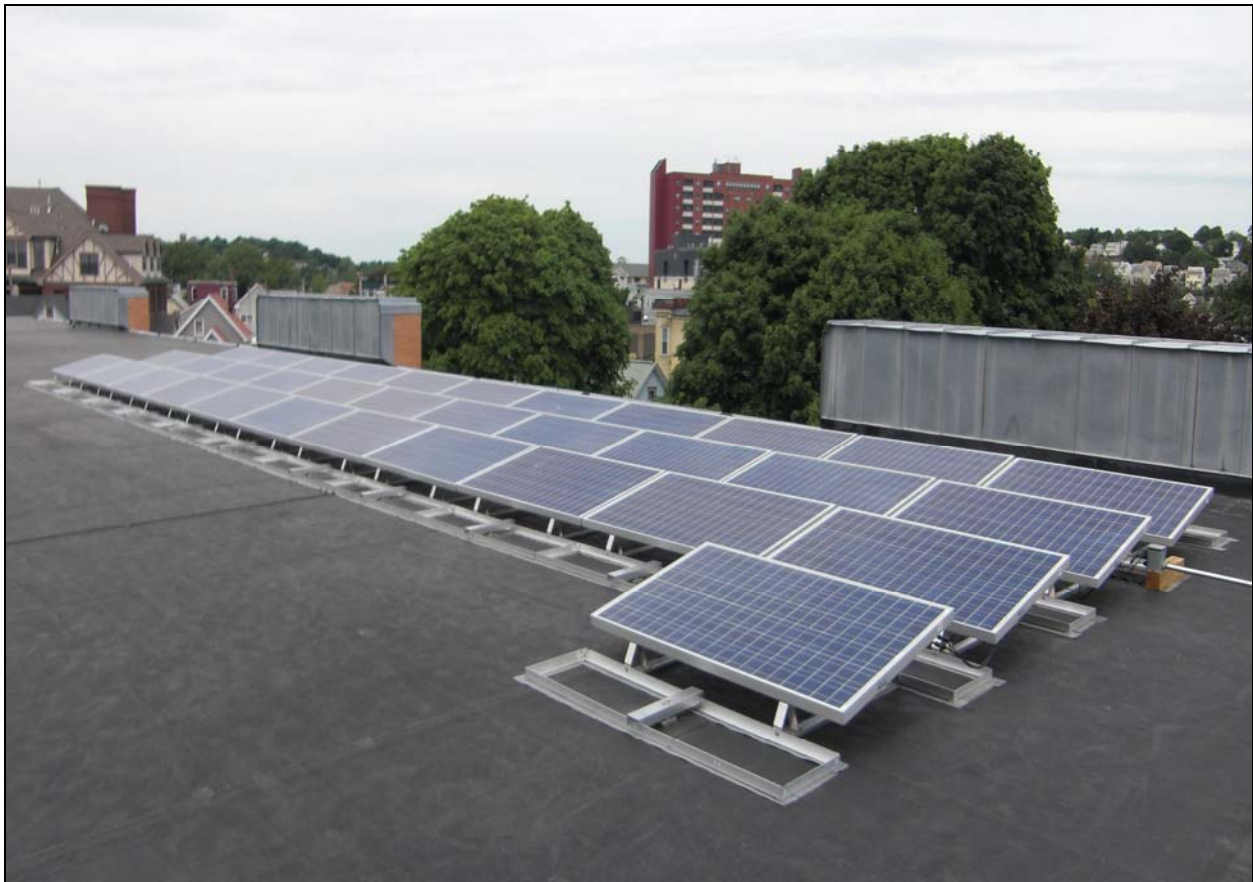
Figure 6: Example of a Roof-Mounted Solar PV System
