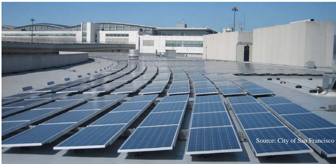
Figure 25: Rooftop Solar Project on San Francisco's Terminal 3
