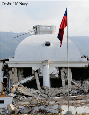
Figure 6-1: The Collapsed Presidential Palace of Haiti
