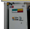
Pilz PLC installed on the cabinet of the PSS of the RF lab
