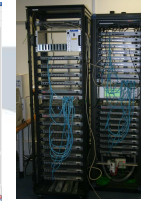
Liberas installed in the Electronics Lab
