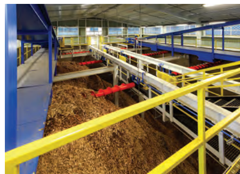
ORNL's new biomass-fired steam plant demonstrates the lab's commitment to renewable energy. (Photo: Jason Richards)
