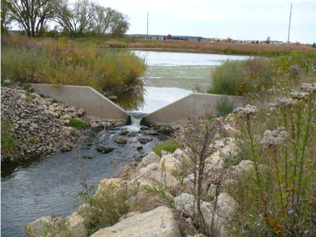
Figure 2. Confluence Pond on Pheasant Branch in Middleton, Wis., in 2008, with a view of the outlet structure. (Photo by W.A. Gebert)
