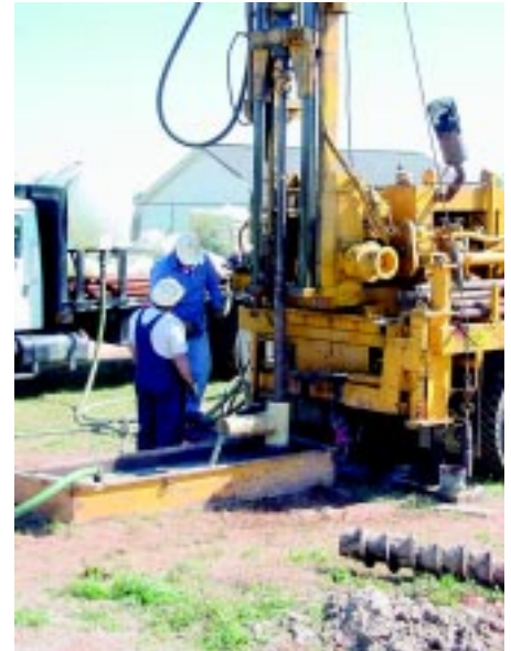
Figure 6. Research well being drilled near Raleigh. Data collected from this and other wells are used to describe the fractured rock aquifer system beneath much of the North Carolina Piedmont, and to understand ground-water movement in this system.
