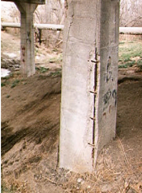
Figure 1. Corrosion-induced deterioration on a bridge column.
