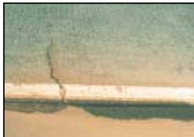
FIGURE 132 Distress Type CRCP 14—Close-up View of Water Bleeding and Pumping
