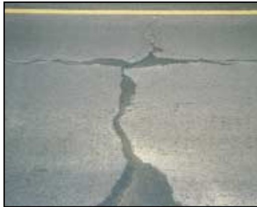
FIGURE 45 Distress Type ACP 15—Water Bleeding and Pumping
