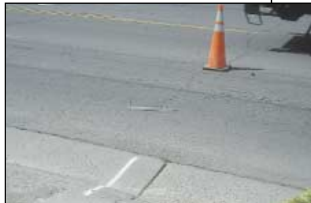
FIGURE 20 Distress Type ACP 6—Moderate Severity Transverse Cracking
