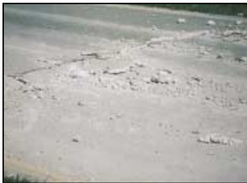
FIGURE 107 Distress Type CRCP 7—A Blowup
