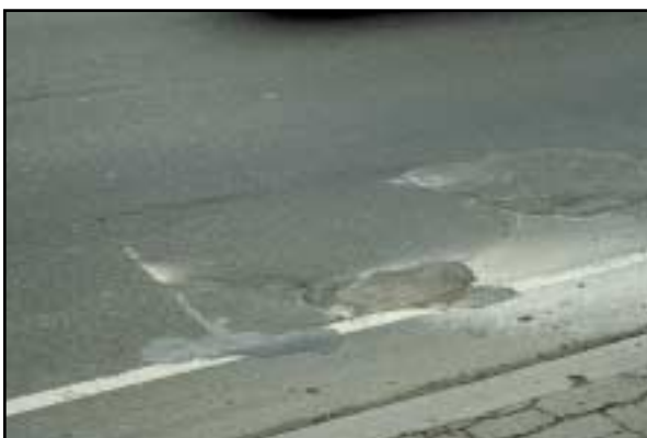
FIGURE 25 Distress Type ACP 7—High Severity Patch
