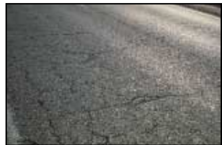
FIGURE 10 Distress Type ACP 2—High Severity Block Cracking
