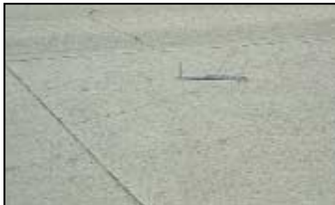
FIGURE 49 Distress Type JCP 1—Low Severity Corner Break
