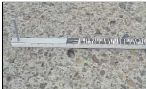
FIGURE 105 Distress Type CRCP 6—Popouts
