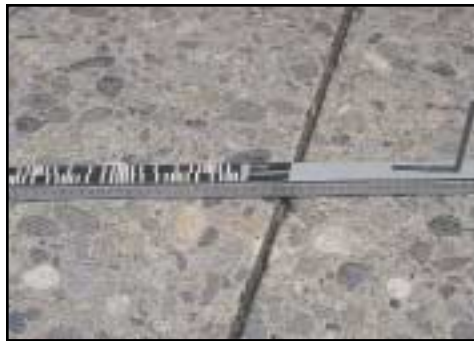
FIGURE 133 Distress Type CRCP 15—Longitudinal Joint Seal Damage
