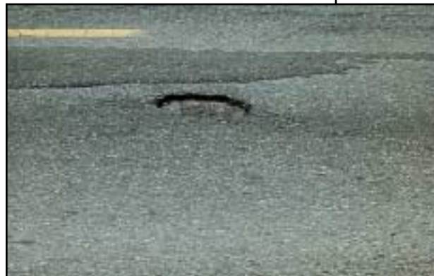
FIGURE 28 Distress Type ACP 8—Moderate Severity Pothole
