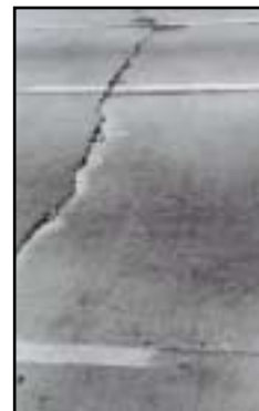
FIGURE 78 Distress Type JCP 12—Faulting of Transverse Cracks
