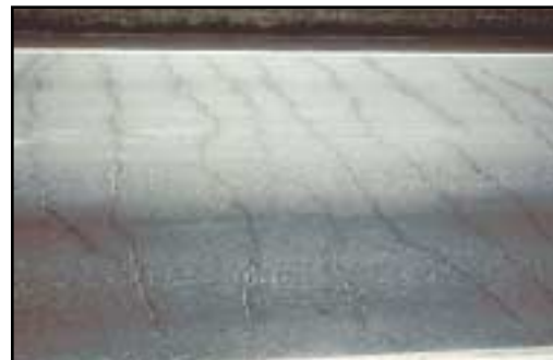
FIGURE 97 Distress Type CRCP 3—Transverse Cracking Pattern
