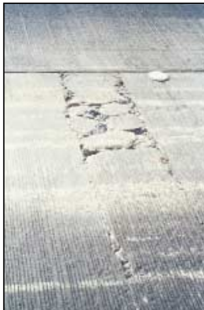
FIGURE 126 Distress Type CRCP 12—High Severity Punchout
