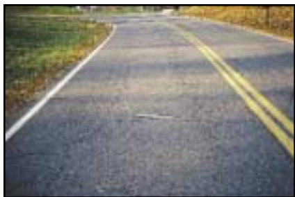
FIGURE 9 Distress Type ACP 2—Block Cracking with Fatigue Cracking in the Wheel Paths
