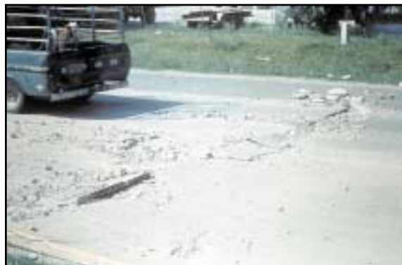
FIGURE 76 Distress Type JCP 11—A Blowup
