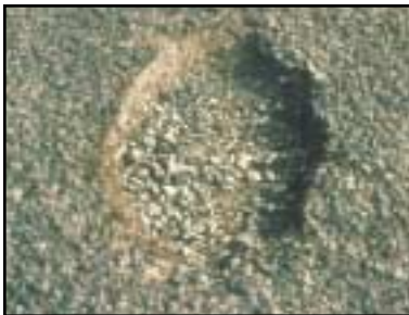
FIGURE 29 Distress Type ACP 8—Moderate Severity Pothole, Close-up View
