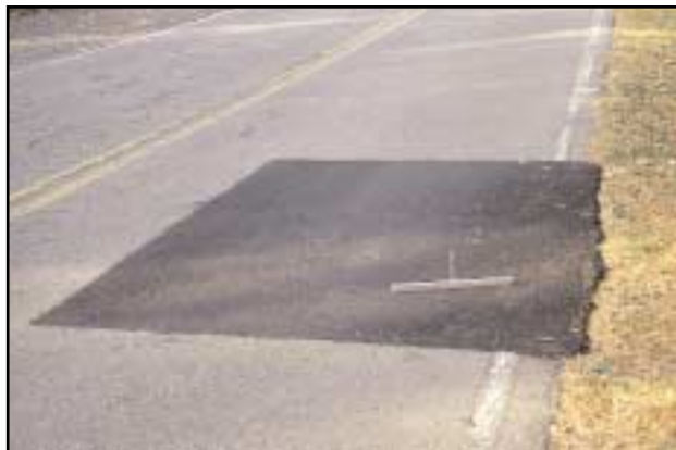
FIGURE 24 Distress Type ACP 7—Moderate Severity Patch
