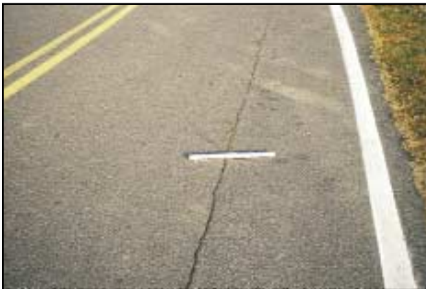
FIGURE 14 Distress Type ACP 4a—Moderate Severity Longitudinal Cracking in the Wheel Path
