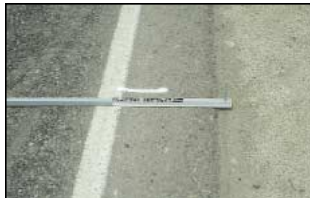
FIGURE 44 Distress Type ACP 14—Lane-to-Shoulder Dropoff
