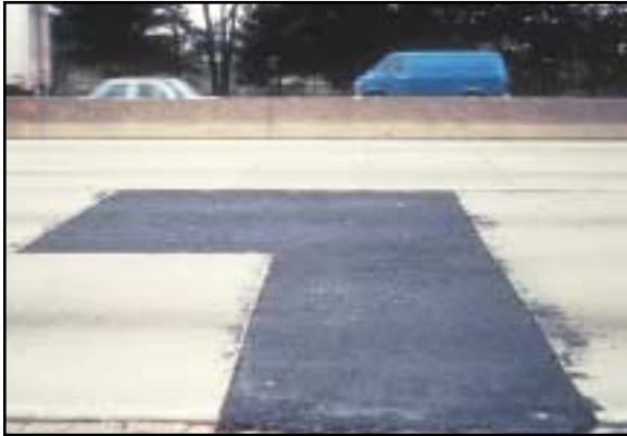
FIGURE 86 Distress Type JCP 15—Large, Low Severity Asphalt Concrete Patch
