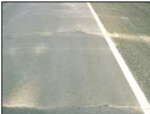
FIGURE 46 Distress Type ACP 15—Fine Material Left on Surface by Water Bleeding and Pumping
