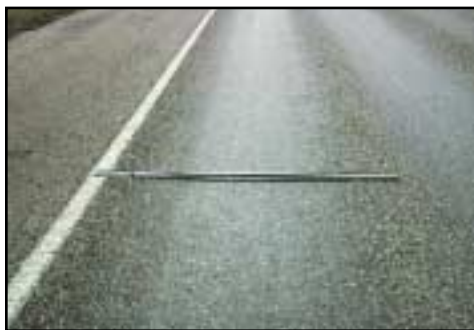
FIGURE 32 Distress Type ACP 9—Rutting
