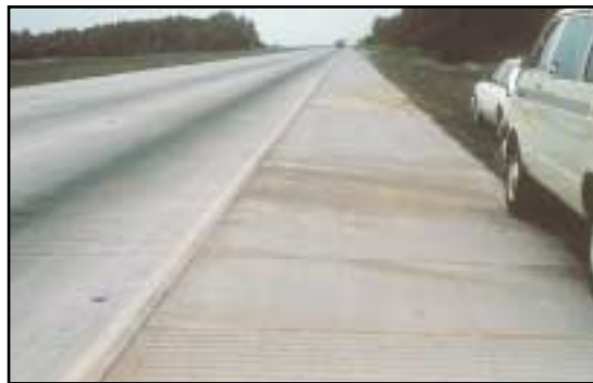
FIGURE 131 Distress Type CRCP 14—Water Bleeding and Pumping
