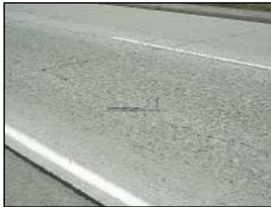
FIGURE 56 Distress Type JCP 3—Moderate Severity Longitudinal Cracking
