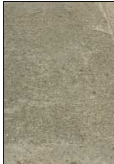
FIGURE 102 Distress Type CRCP 4b—Scaling
