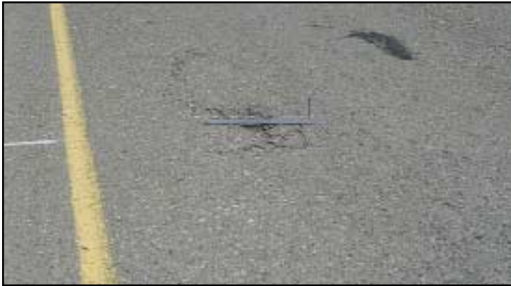
FIGURE 27 Distress Type ACP 8—Low Severity Pothole
