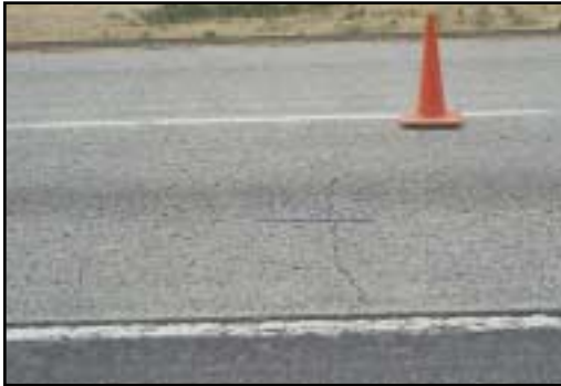
FIGURE 98 Distress Type CRCP 3—Low Severity Transverse Cracking
