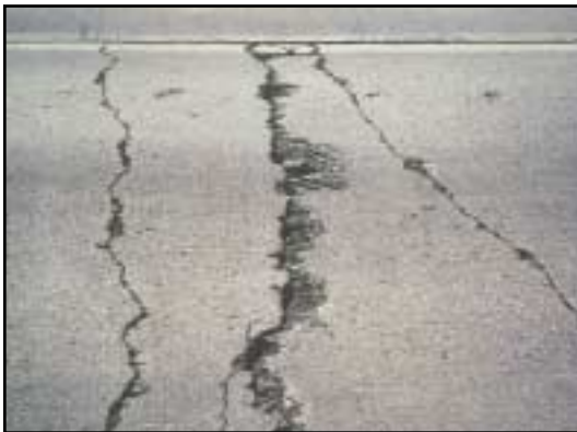
FIGURE 100 Distress Type CRCP 3—High Severity Transverse Cracking
