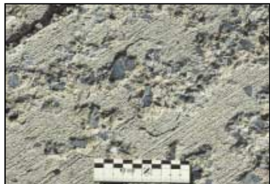
FIGURE 71 Distress Type JCP 8b—Scaling, Close-up View
