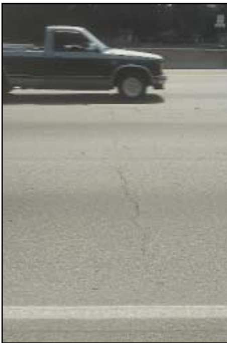
FIGURE 19 Distress Type ACP 6—Low Severity Transverse Cracking
