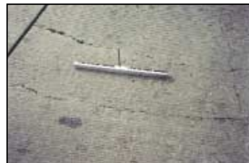
FIGURE 124 Distress Type CRCP 12—Low Severity Punchout
