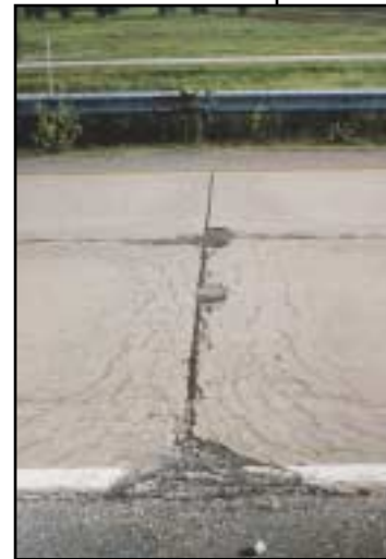
FIGURE 53 Distress Type JCP 2—High Severity “D” Cracking with Loose and Missing Material
