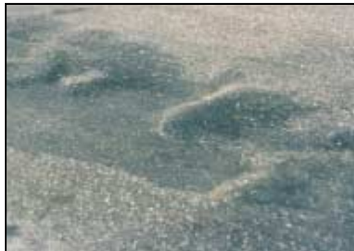
FIGURE 35 Distress Type ACP 10—Shoving in Pavement Surface
