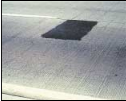
FIGURE 120 Distress Type CRCP 11—Low Severity Asphalt Concrete Patch
