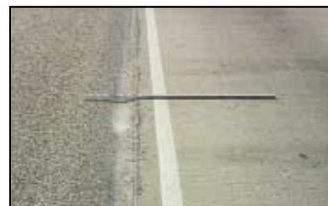
FIGURE 115 Distress Type CRCP 9—Lane-to-Shoulder Dropoff
