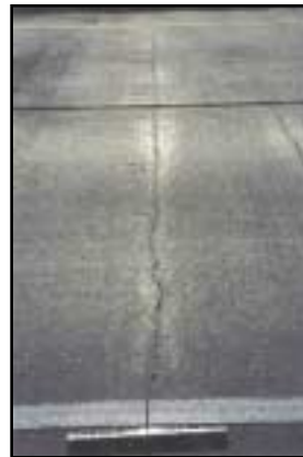
FIGURE 113 Distress Type CRCP 8— Low Severity Transverse Construction Joint Deterioration
