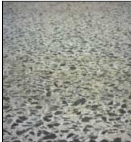
FIGURE 103 Distress Type CRCP 5—Polished Aggregate
