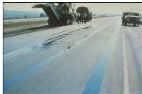
FIGURE 33 Distress Type ACP 9—Standing Water in Ruts
