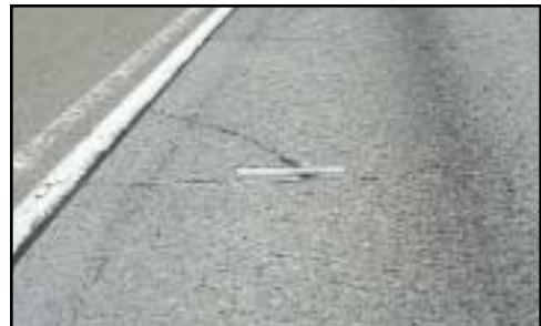
FIGURE 50 Distress Type JCP 1—Moderate Severity Corner Break
