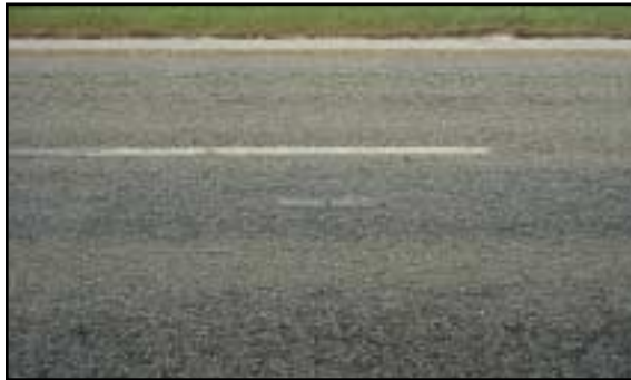
FIGURE 36 Distress Type ACP 11—Discoloration
