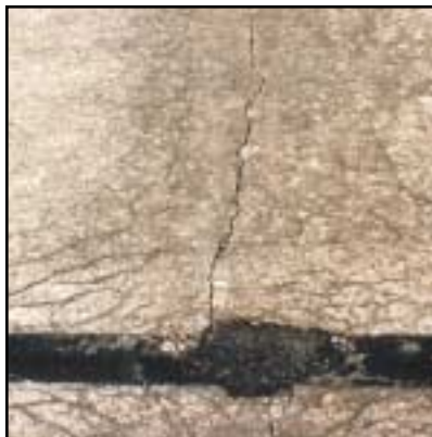
FIGURE 91 Distress Type CRCP 1—Moderate Severity “D” Cracking at Transverse Crack
