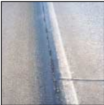
FIGURE 82 Distress Type JCP 14—Poorly Sealed Lane-to-Shoulder Separation
