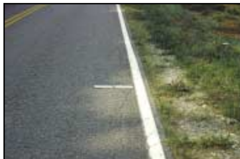
FIGURE 12 Distress Type ACP 3—Low Severity Edge Cracking
