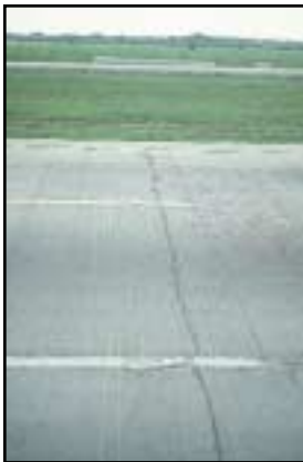
FIGURE 112 Distress Type CRCP 8— Moderate Severity Transverse Construction Joint Deterioration
