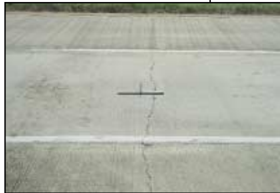
FIGURE 99 Distress Type CRCP 3—Moderate Severity Transverse Cracking
