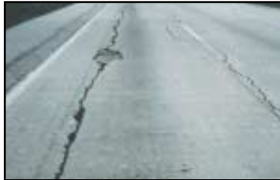
FIGURE 95 Distress Type CRCP 2—High Severity Longitudinal Cracking
