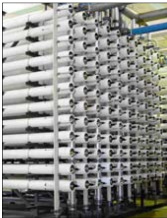
Reverse osmosis membrane modules at the Larnaca desalination plant, Cyprus. Photo courtesy of Thomas Pankratz.
