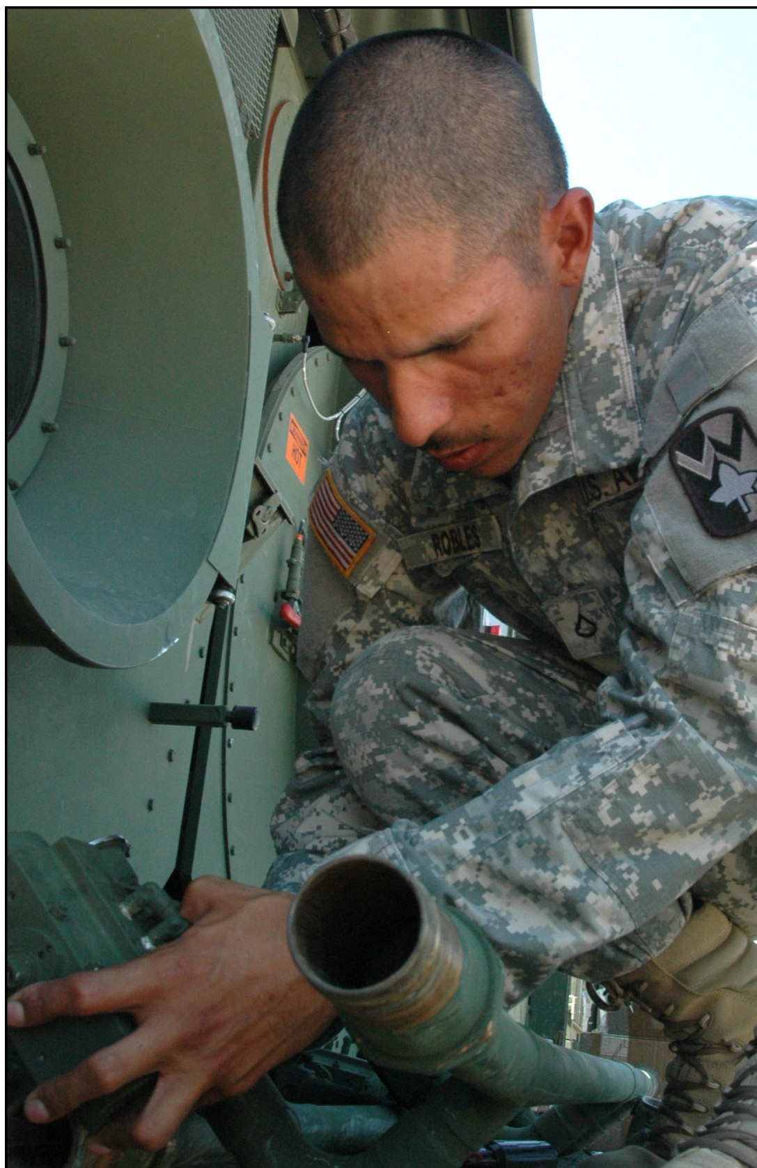
Pfc. Raul Robles, 157th Quartermaster Company, replaces ball valves that substitutes for the input and output valves of a laundry advanced system.
