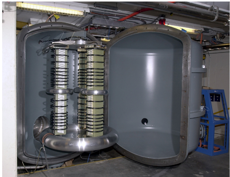
FEL High Voltage Power Supply
