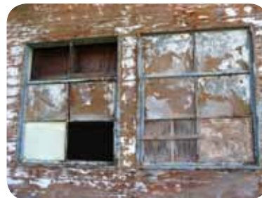
Peeling lead-based paint
