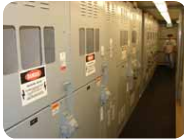
Electrical switch gear
