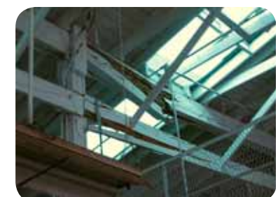
Termite damage to structural roof members of historic Machine Shop
