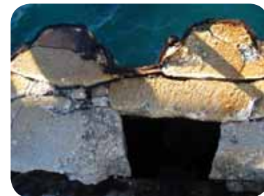
Deteriorated bulkhead on Inner Harbor
