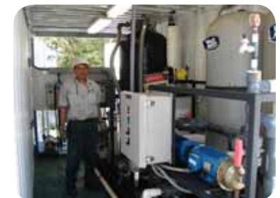
Water treatment facility
