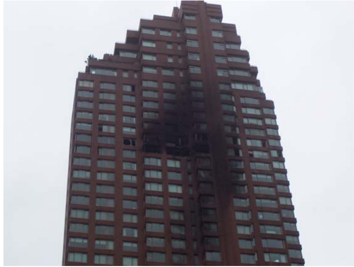
Figure 7. Photo of Belaire Condominium after being hit by the Lidle aircraft
