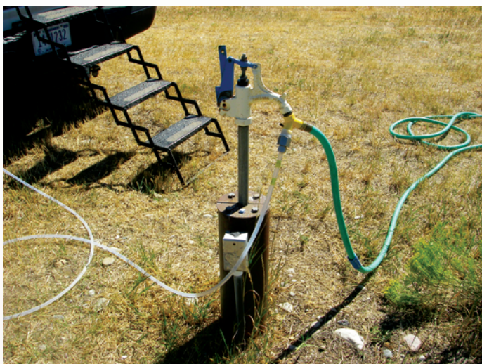
Figure 3. Wellhead connections for groundwater sampling that lead to the mobile water-quality laboratory and discharge line.
