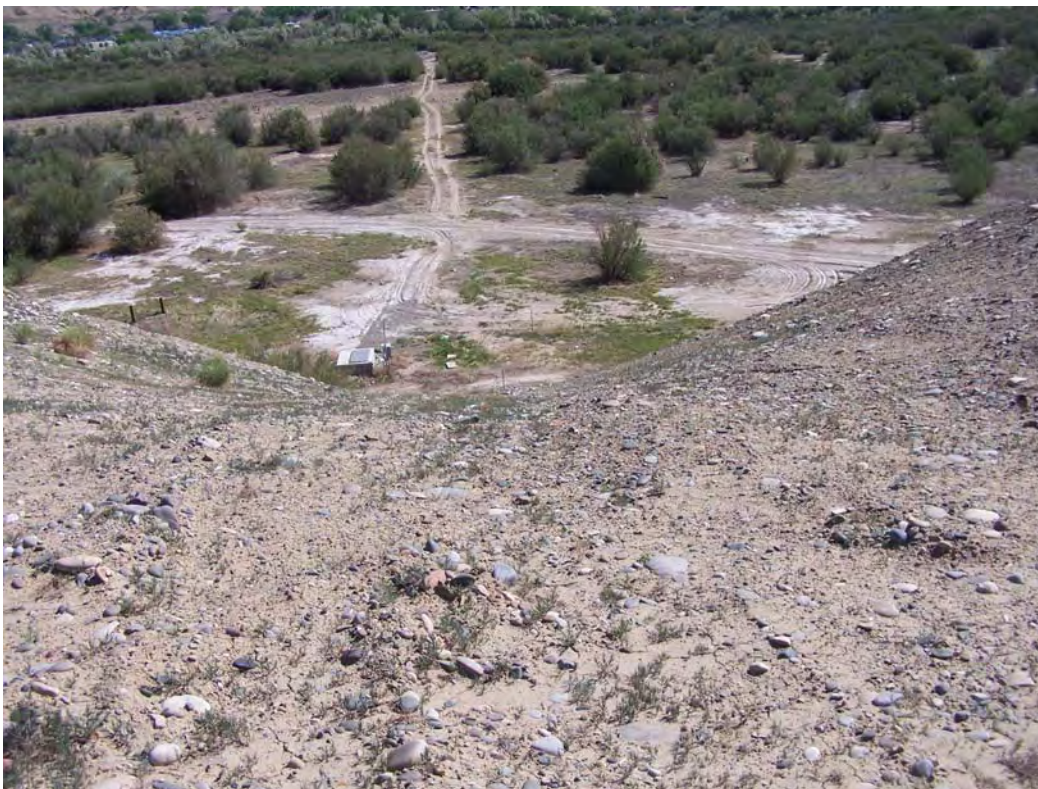
SHP 5/08. PL-3. View from top of escarpment of erosion area below berm near SM-1; no new erosion is evident.
