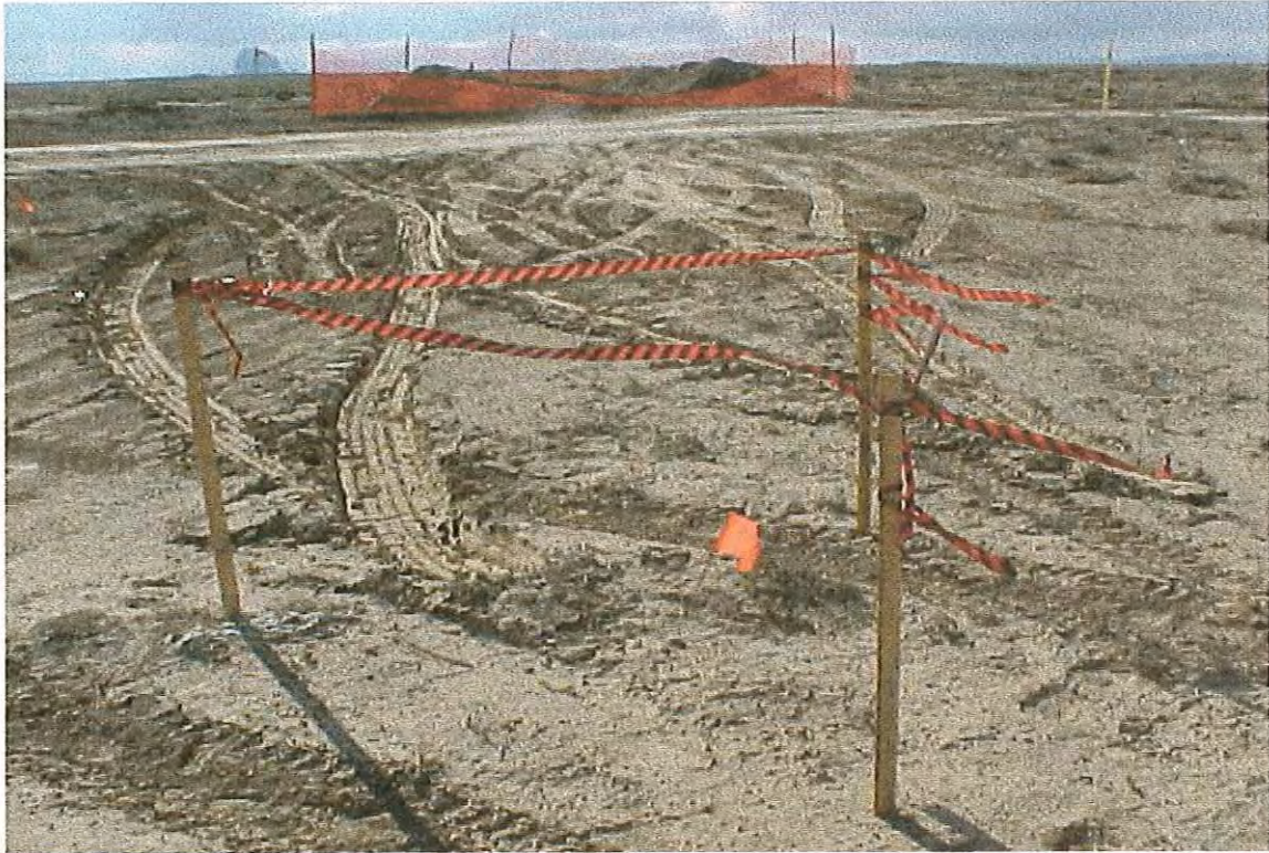
Photograph 4: Water truck turn around area at SMSC Many Devil's Wash construction site looking west. Permitted ROW is located in background where a drain site is fenced with orange visqueen.
