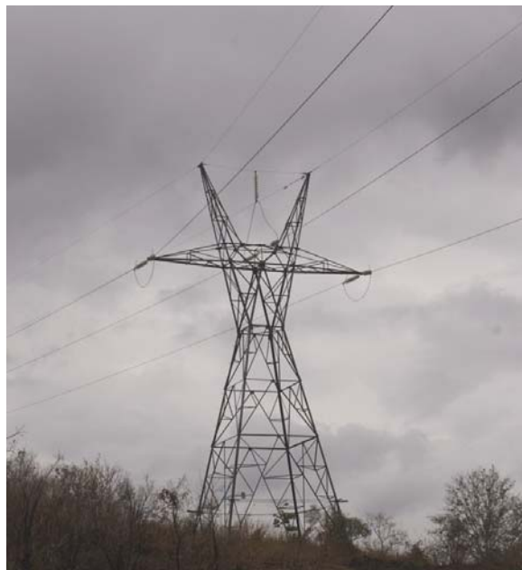
A 132kV TANESCO transmission line. Having diversified to sources beyond hydro, Tanzania has sufficient generation of power at the moment, but suffers from antiquated and insufficient transmission and distribution systems.
