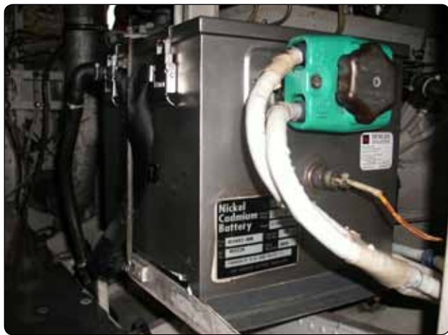
Figure 9-34. NiCd battery installation.
