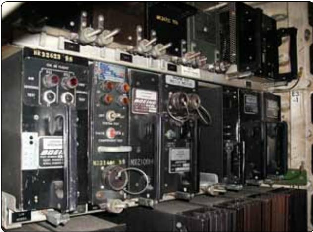
Figure 9-81. Line replaceable units in an equipment rack.
