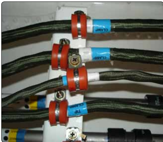
Figure 9-133. Positive separation of wire and fluid lines and wire clamps.
