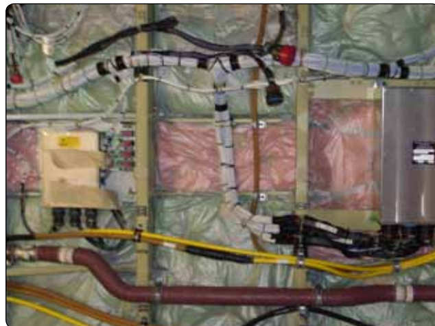
Figure 9-111. Shielded wire harness.
