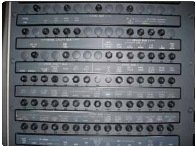
Figure 9-173. Circuit breaker panel.
