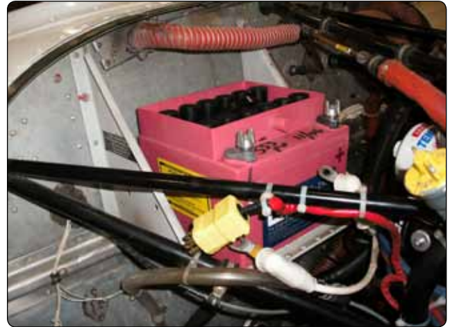
Figure 9-32. Lead acid battery installation.
