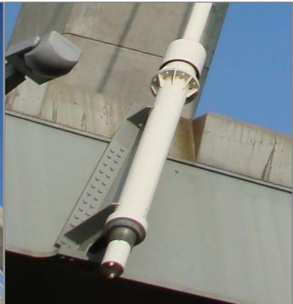
C. Close-up of anchor plate securing cable to a steel girder. According to the Phase I report, six of the anchor plates are deformed.
