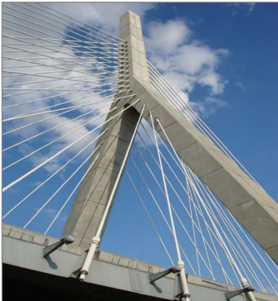
B. Close-up of cables
