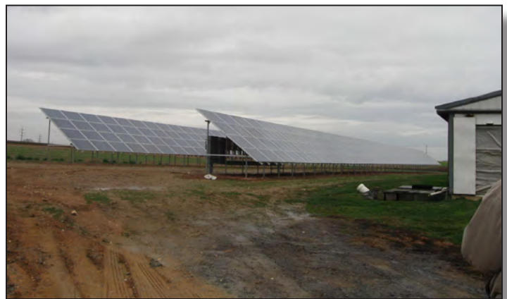
A 75 kW photovoltaic system offsets grid-purchased electricity for a small hog farm with additional beef and tobacco operations.
