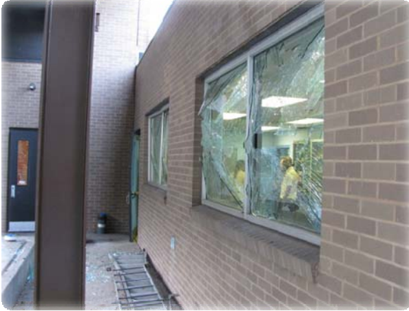
Windows damaged from the explosion.
