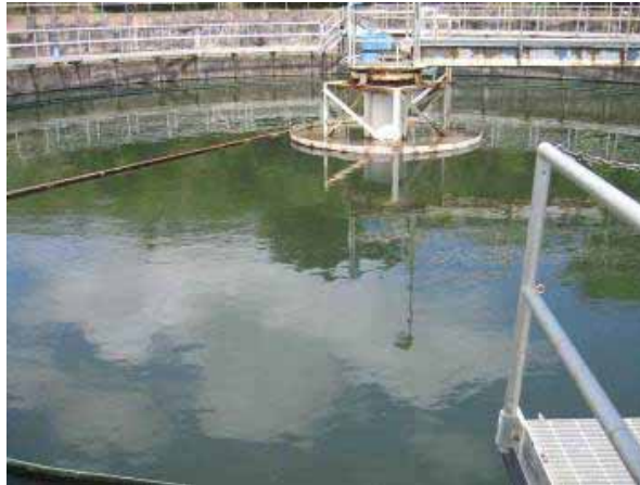
Figure 6-14 Primary tank, Saipan sewage treatment facility
