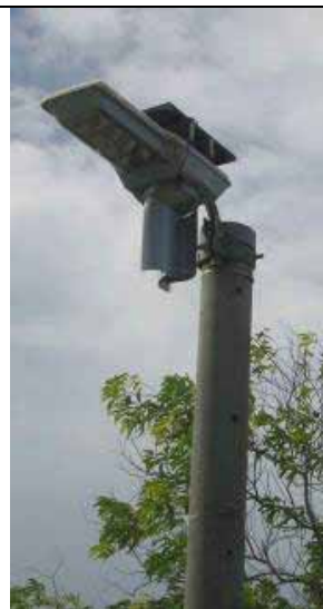
Figure 13-15—Solar/Wind Powered Streetlight on Babeldaob for trial
