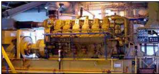
Generator Unit No. 7
