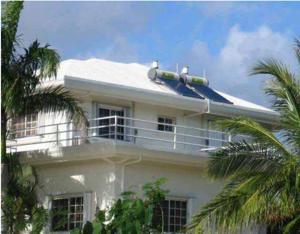
Figure 6-13 Home with Chinese solar water heater installation
