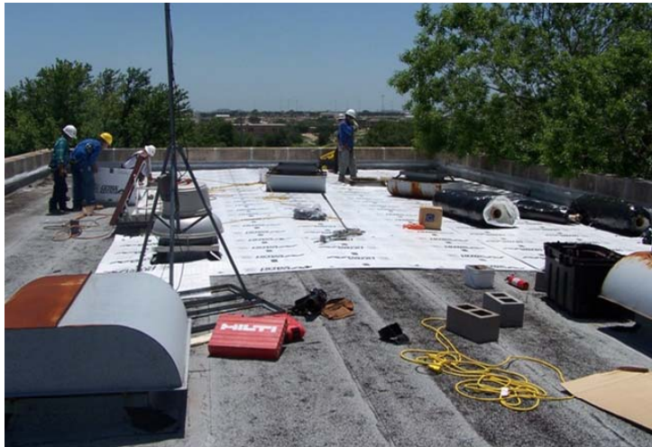
Contractors roll the insulation onto the roof of building 29014, which can be accomplished in almost half the time as placing traditional asphalt shingles.
